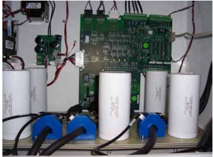
Inverters have capacitors that store energy which is discharged soon after power to the inverters is disconnected.
