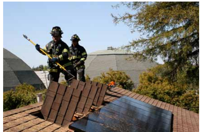
Firefighters need to practice and train for roof operations and ventilation techniques when photovoltaic systems are present.
