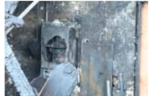
A content fire in the garage of this residence destroyed the PV inverter box.
